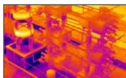
Electric Equipment Inspection
